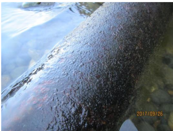
Photo C-41. Minor surface corrosion on DIP at wet/dry zone
