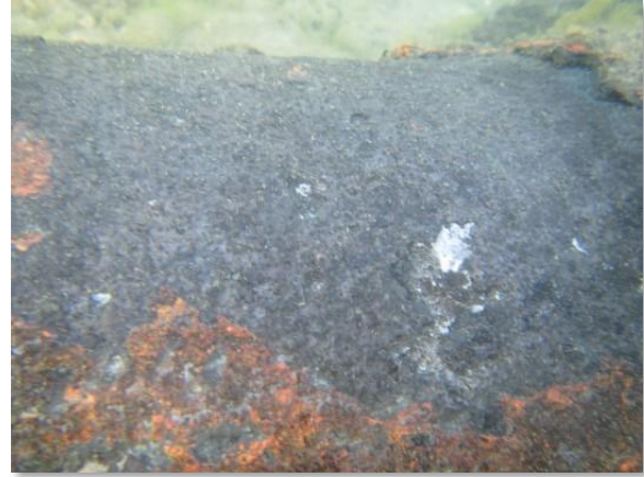
Photo C-44. Pipe surface underneath corrosion layer
