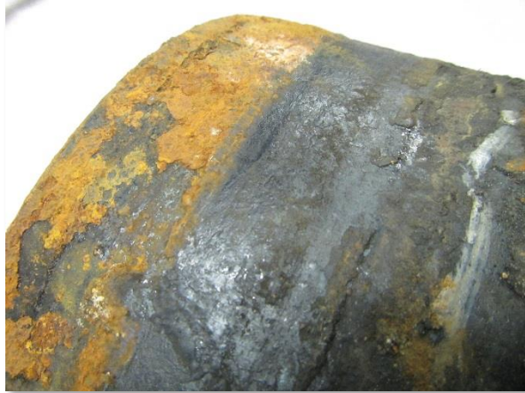
Photo 3-11. Corrosion on spigot end of pipe exposed to water inside joint (left); relatively clean strip under gasket (center).
