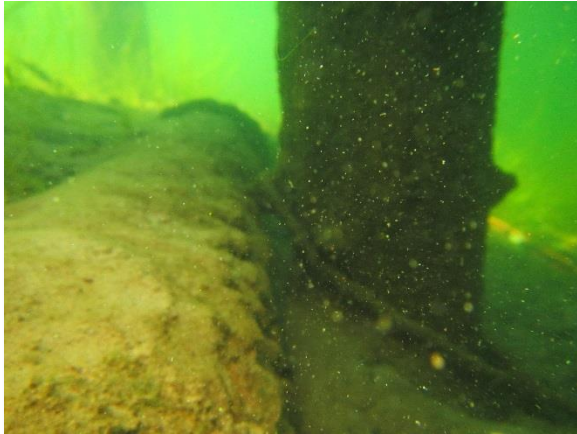
Photo 2-11. Lakeline sits only inches from dock piling near 3719 and 3805 Lake Washington Blvd. North
