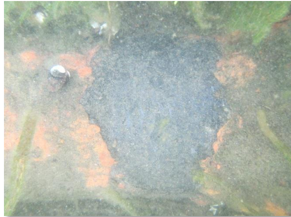
Photo 2-21. Corrosion on lateral at 3717 Lake Washington Blvd. North
