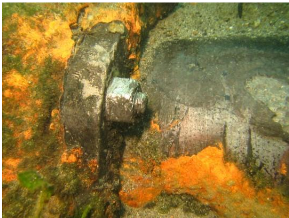
Photo C-58. Pipe and joint surface after removal of corrosion products
