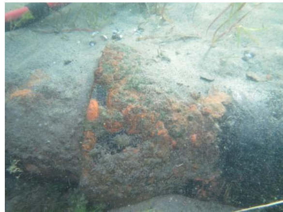
Photo C-50. Bell/spigot joints with corrosion, but in fair condition
