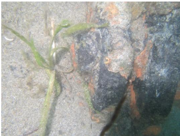
Photo C-49. Nuts, bolts glands of mechanical joints with corrosion but in fair condition
