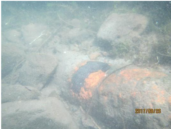
Photo C-15. Corrosion scale/tuberculation; large rocks around pipe
