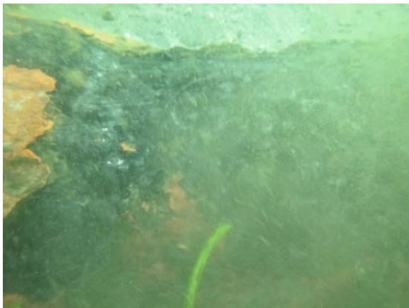
Photo C-35. Surface of pipe after corrosion scale/tuberculation was removed
