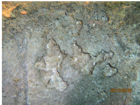
Photo C-22. Pitted surface; up to 0.06-inch-deep pits
