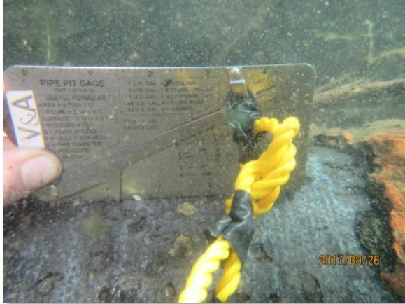
Photo C-17. Pitting up to 0.06 inches deep
