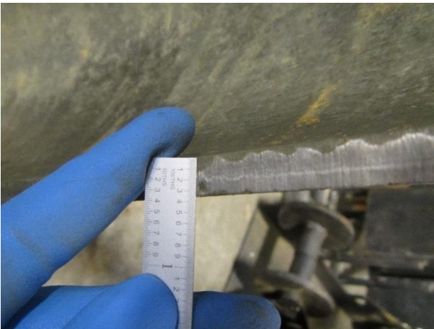
Figure 6.3-2 Graphitization on Interior Surface of Manhole 4 Sample
