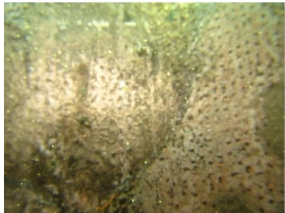
Photo C-65. Dimple pattern on pipe surface (DIP)
