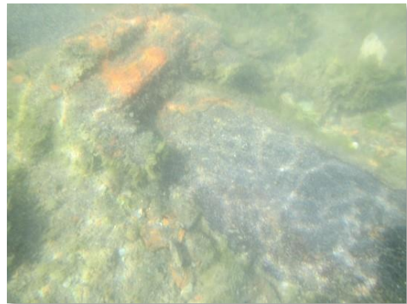
Photo C-46. Mechanical joint (second from shore) with surface corrosion on gland ring
