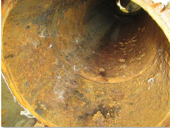
Photo 3-5. Corroded surfaces near joint of Manhole 5 sample; lining failed around joint.
