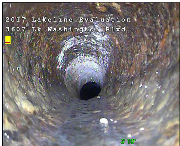
Photo 2-24. Staining on lateral interior
