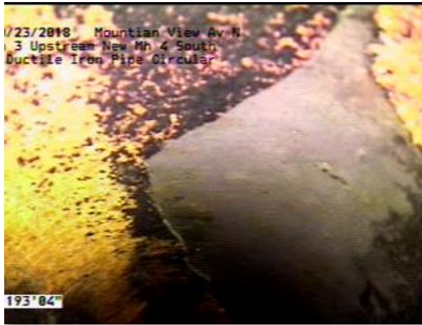
Photo 3-13. Typical lining delamination with smooth metal surface behind.
