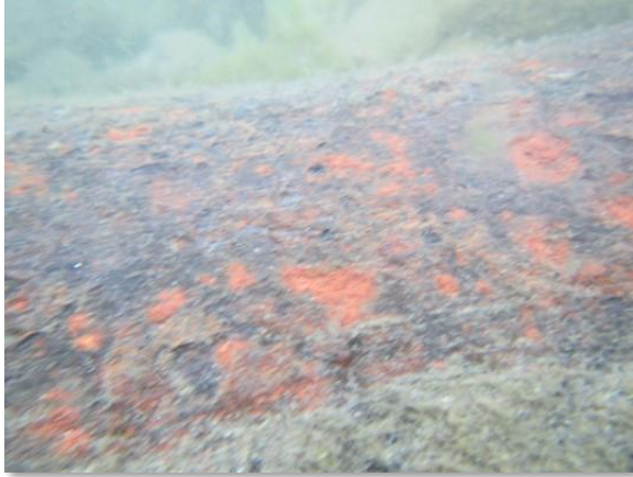
Photo C-43. Surface corrosion on DIP
