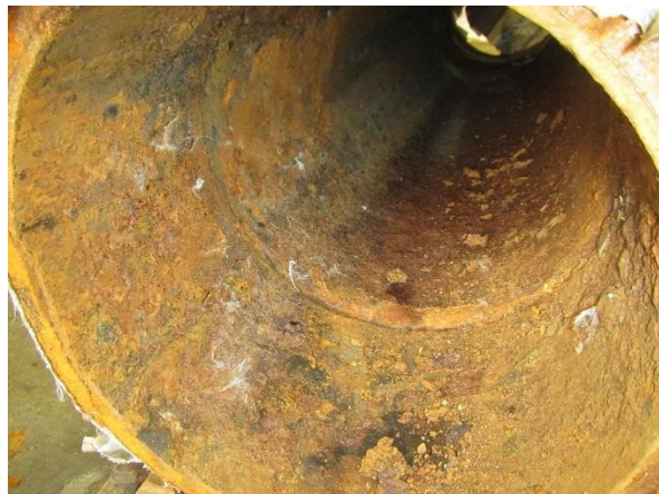
Figure 6.3-5 Corroded Surfaces near Joint of Manhole 5 Sample; Lining Failed around Joint
