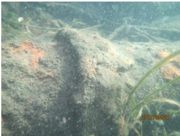
Photo C-19. Bell/spigot joint on south end of exposed reach
