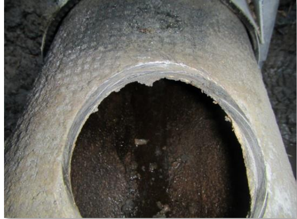
Photo C-10. Pipe coupon hole
