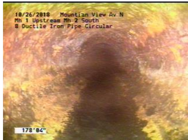
Photo 3-16. Typical moderate to significant corrosion at high points (brown area).
