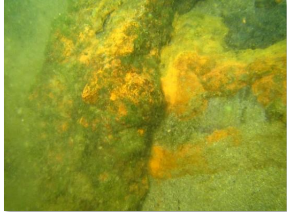
Photo C-57. Corrosion scale/tuberculation near mechanical joint gland and bolts
