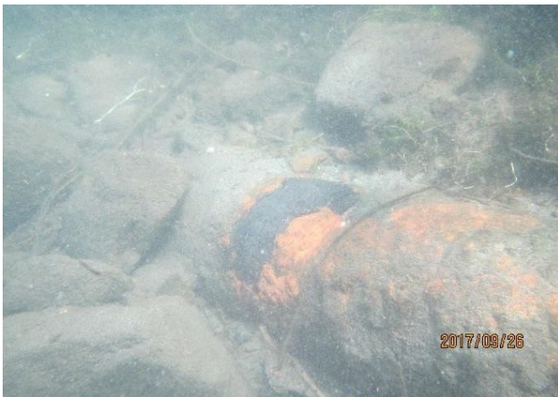
Figure 6.1-2 Area of Scaling and Tuberculation on Mainline; Large Rocks Around Mainline at 2811 Mountain View Avenue North
