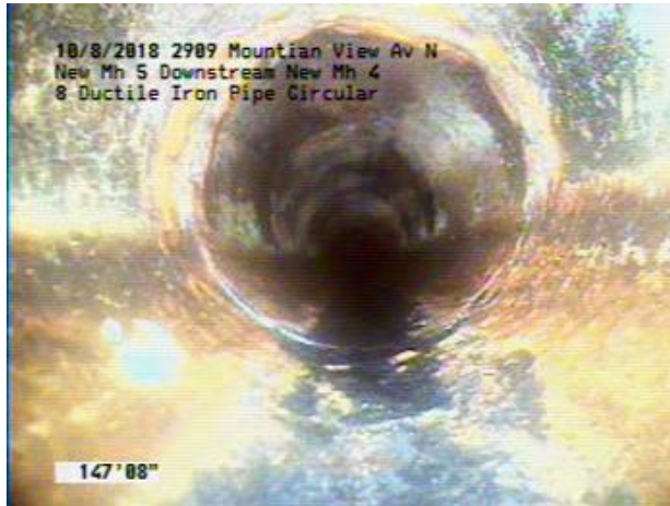
Photo 3-17. Typical corrosion deposits at joint.
