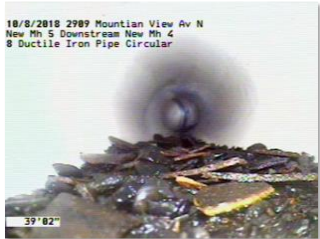
Photo 3-14. Debris and sediment, some of which appears to be chunks of cement mortar lining material.
