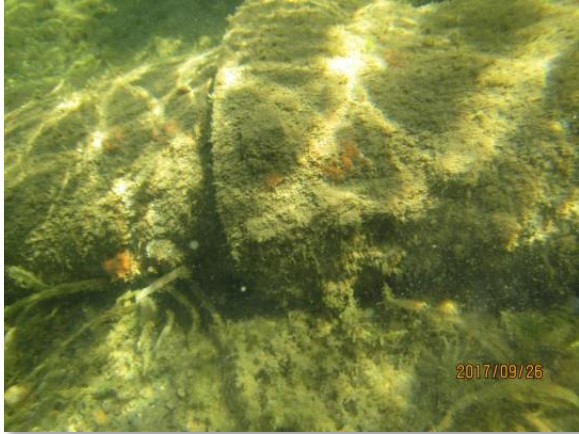
Photo C-29. Bell/spigot joint covered in dirt/debris
