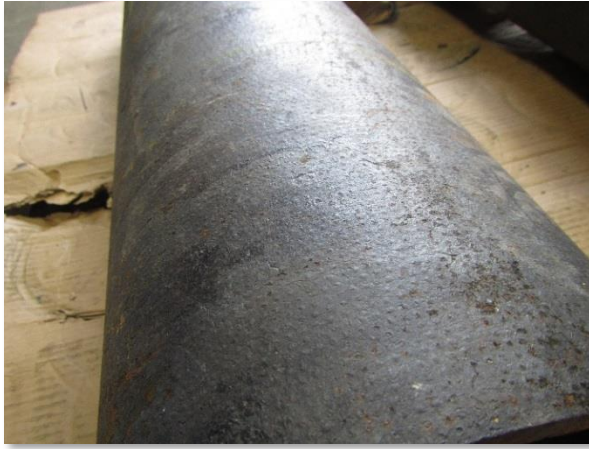
Photo 3-1. Typical dimple pattern on mainline samples and coupon; however, this is not ductile iron pipe.
