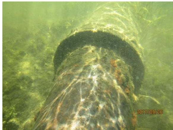
Photo C-32. Corrosion tubercles underneath dirt/debris layer near bell/spigot joint
