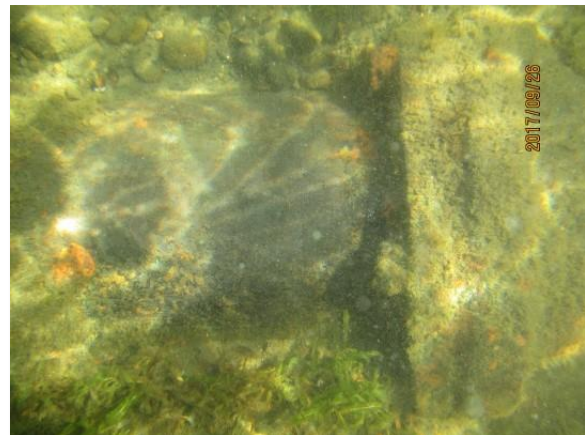
Photo C-28. Top view of mechanical joint
