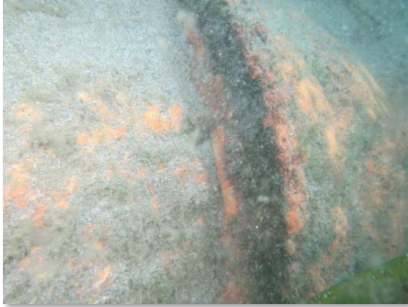
Photo C-37. Corrosion scale/tuberculation on bell/spigot joint
