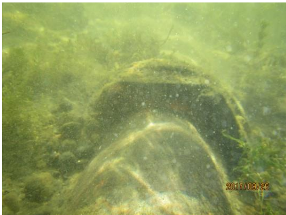
Photo C-27. Mechanical joint at fitting
