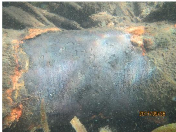
Photo C-20. Pipe surface underneath scale/deposits reach
