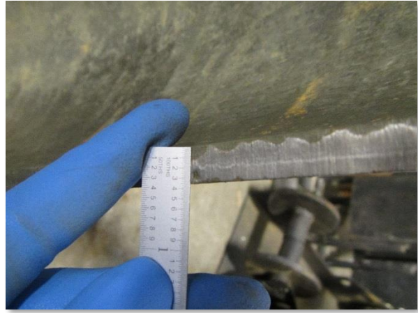
Photo 3-2. Graphitization on interior surface of Manhole 4 sample.
