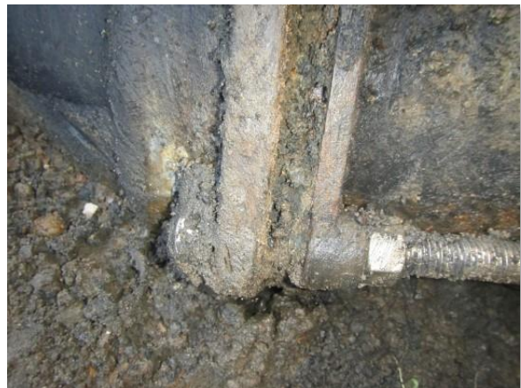
Photo C-8. Stainless steel bolts on mechanical joint
