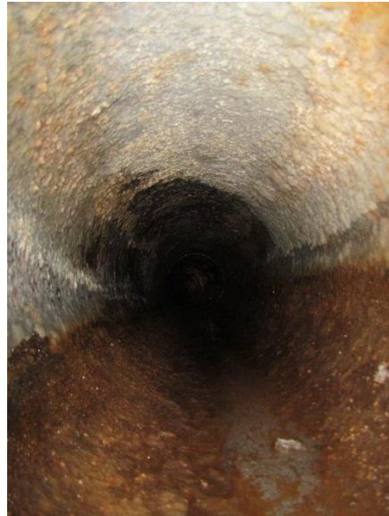
Photo 2-19. Interior of Lakeline looking downstream; appears to be corrosion staining on lower half of pipe
