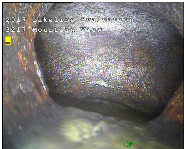
Photo 2-12. Wye or tee fitting connection to mainline at 3217 Mountain View Ave. North
