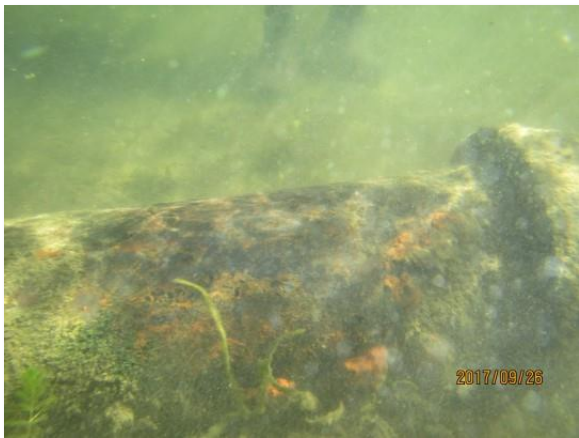
Photo C-31. Corrosion tubercles underneath dirt/debris layer near bell/spigot joint
