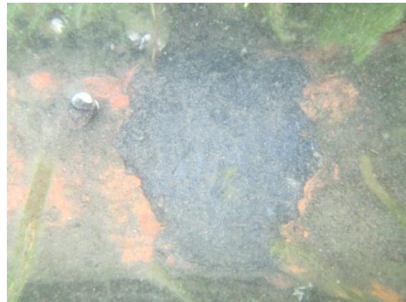
Photo C-53. Corrosion scale/tuberculation; pipe surface after removal of corrosion in fair condition
