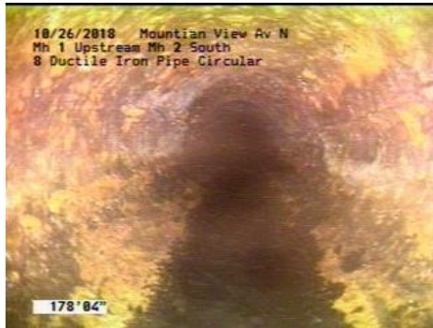
Figure 6.2-4 Typical Moderate to Significant Corrosion at High Points (Brown Area)
