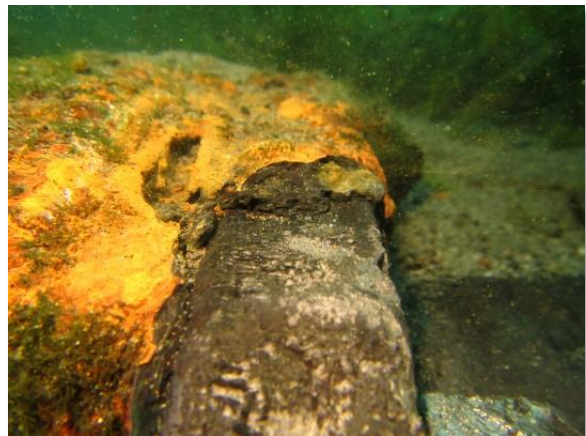
Photo C-61. Corrosion scale/tuberculation on bell/spigot joint
