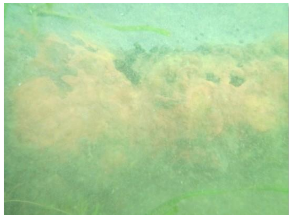
Photo C-34. Corrosion scale/tuberculation on individual pipe segments
