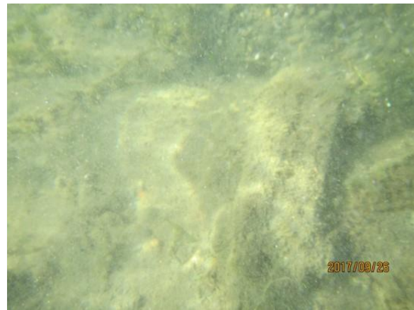
Photo C-26. Mechanical joint for lateral connection partially covered in dirt/debris
