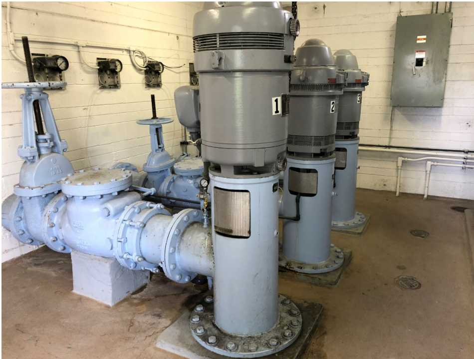
Highlands Booster Pump Station
