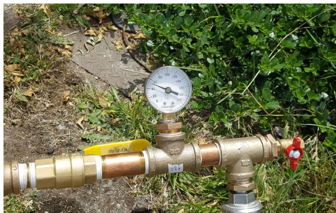
Pressure Recording Equipment used during field testing
