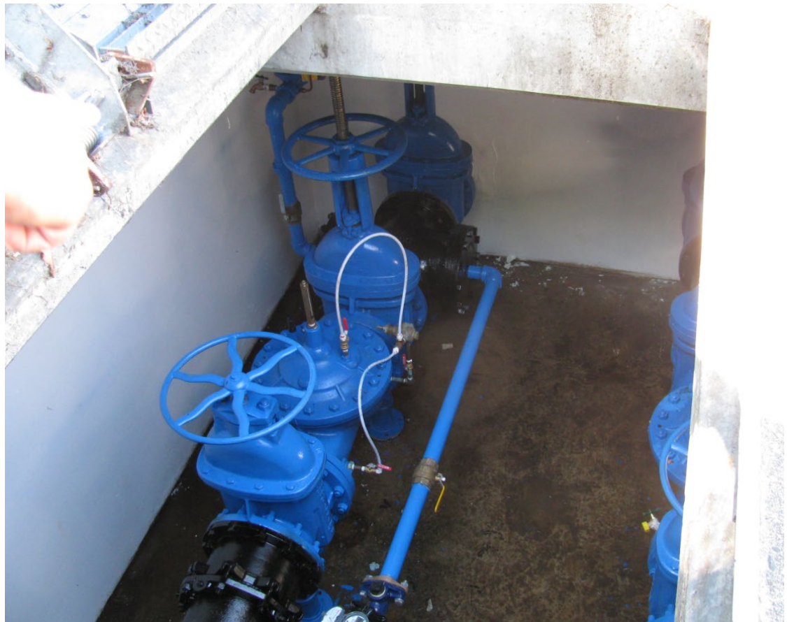
Pressure Reducing Valve (PRV) 52
