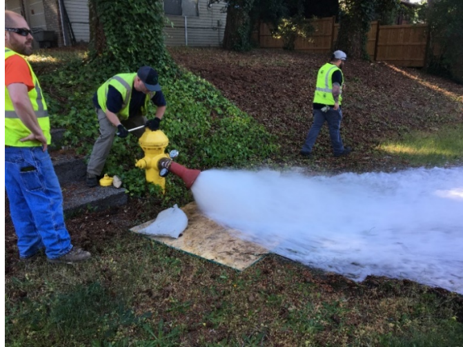
Fire Hydrant Test – June 2018
