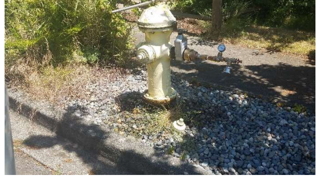
Logger setup for pressure hydrant P1
