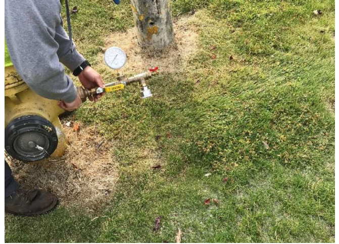
Logger setup for pressure hydrant 1
