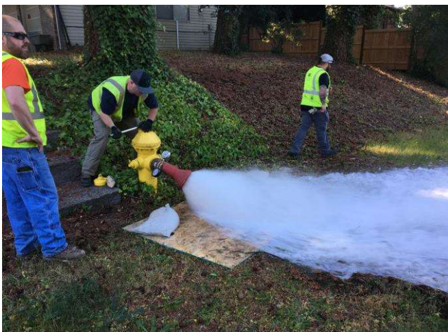
Diffuser setup and flowing the hydrant F1
