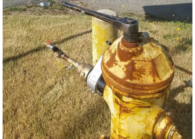
Logger setup for pressure hydrant 1
