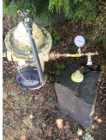
Logger setup for pressure hydrant P2
