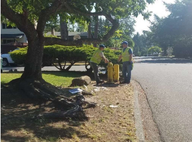
Location of pressure hydrant 1
