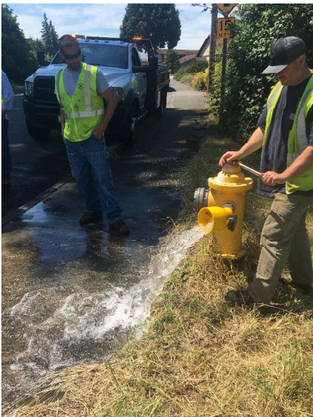
Diffuser of flowing hydrant F1
