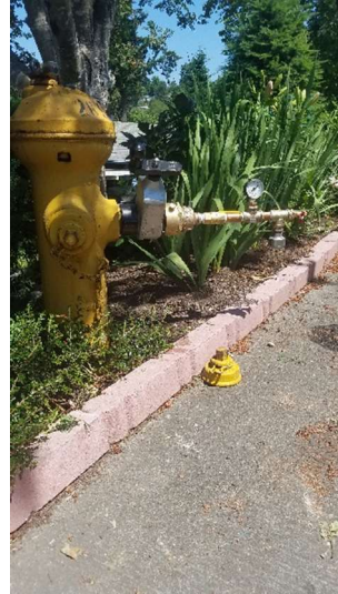
Logger setup for pressure hydrant P1
