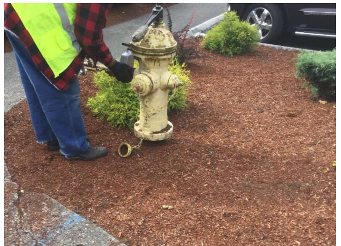
Logger setup for pressure hydrant 2
