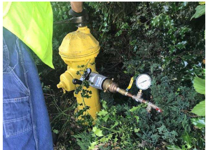
Logger setup for pressure hydrant 2
