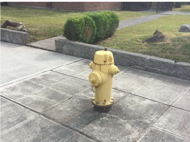
Location of pressure hydrant 2
