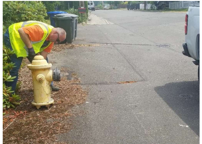
Logger setup for pressure hydrant 1
