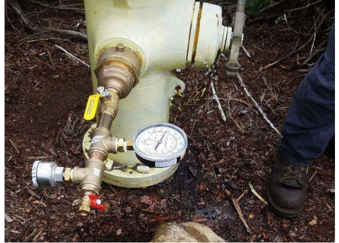
Logger setup for pressure hydrant 1
