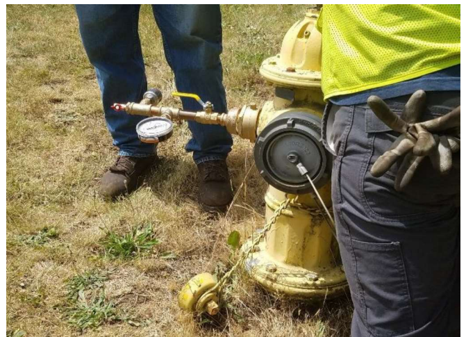
Logger setup for pressure hydrant 2
