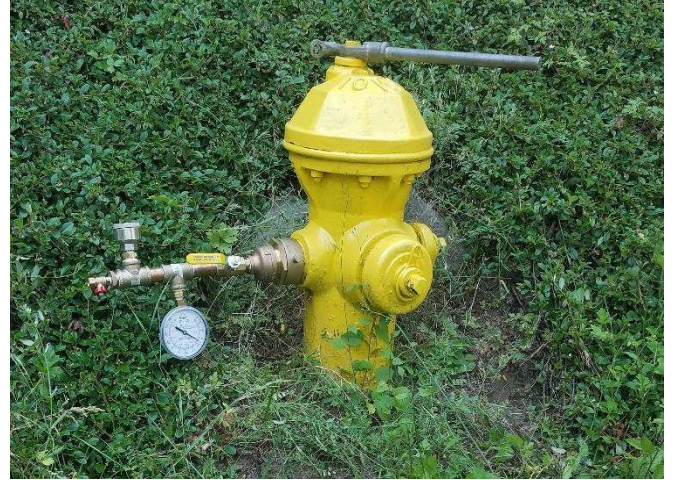
Logger setup for pressure hydrant 1
