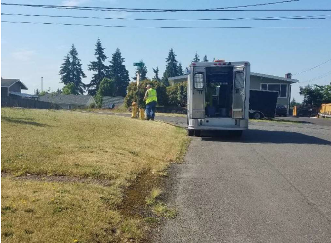
Location of pressure hydrant 1
