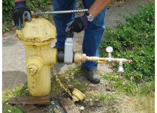
Logger setup for pressure hydrant 1
