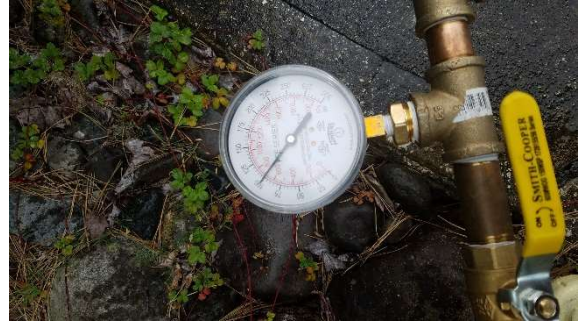
Logger setup for pressure hydrant P1
