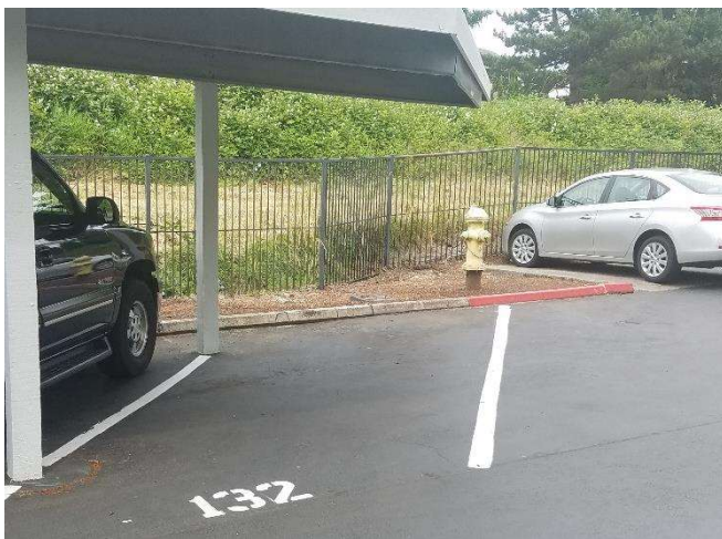
Location of pressure hydrant 2
