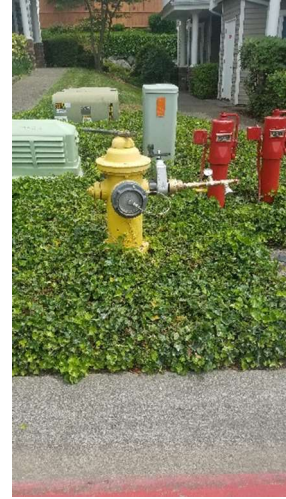
Logger setup for pressure hydrant P1
