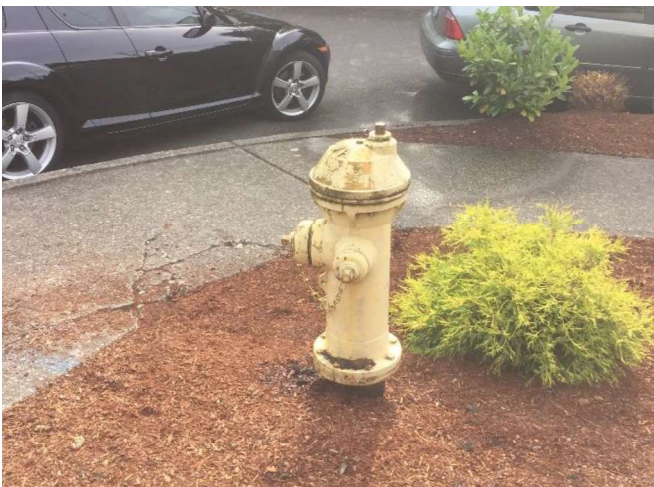
Location of pressure hydrant 2
