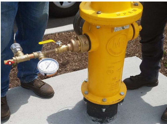
Setup of pressure hydrant 2
