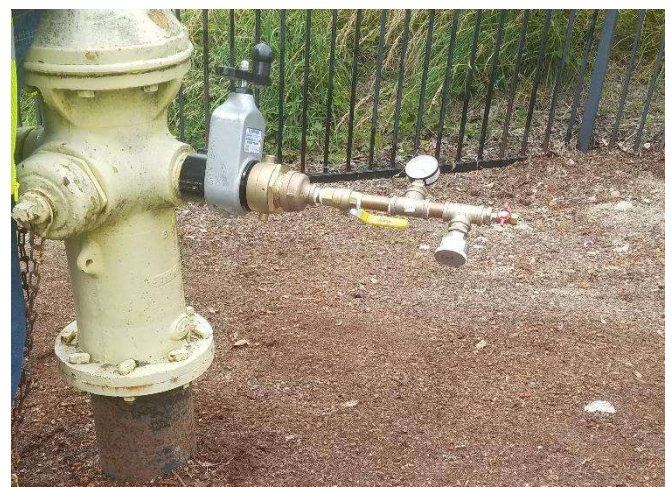
Logger setup for pressure hydrant 2
