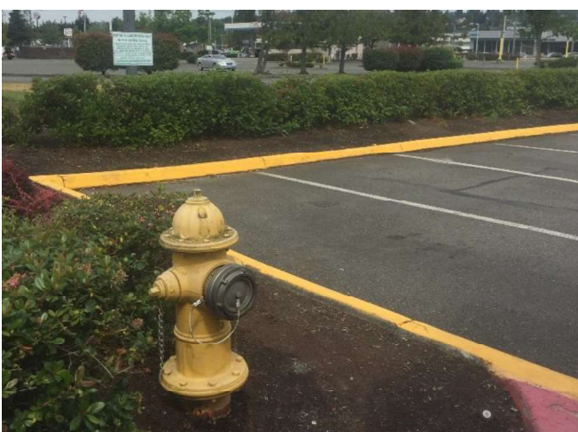
Location of flowing hydrant 2 (F2)
