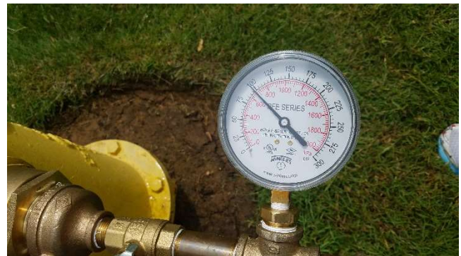
Logger setup for pressure hydrant P2
