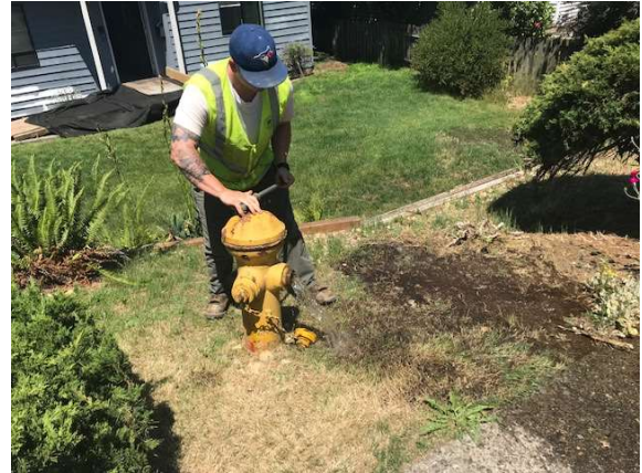
Logger setup for pressure hydrant P2
