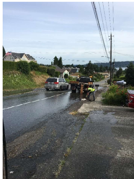
Surrounding area of flowing hydrant F1
